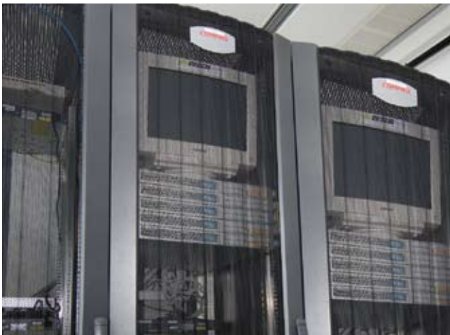
Serverhousing-Center der IKB in Innsbruck
